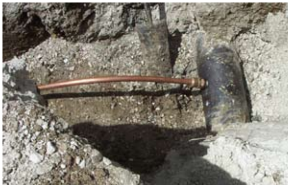
1 inch diameter service connection
