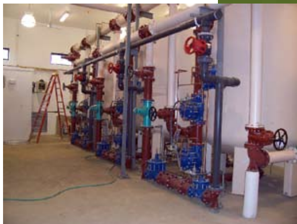
Three 8 foot diameter cation exchange units
