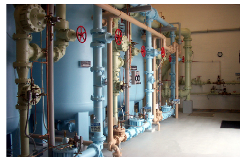
Water Treatment Unit & Piping
